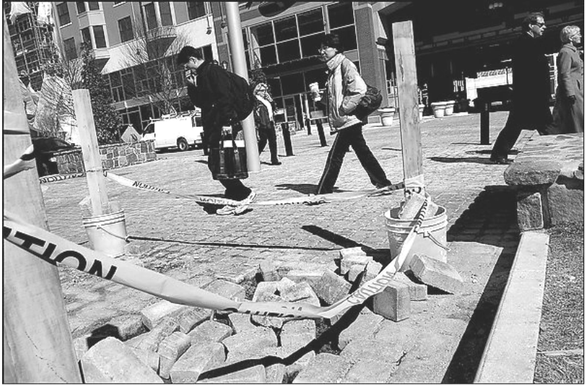
Officials are trying to figure out what caused brick along Maryland Ave and Gibbs St to buckle less than six months after it was laid. Photo Credit: By Lois Raimondo - The Washington Post
